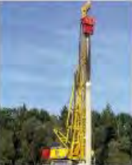
Pletasichs Hydroelectric Weir Structure, Germany
